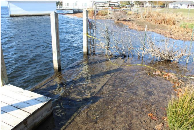
2020 High Water Flooding
